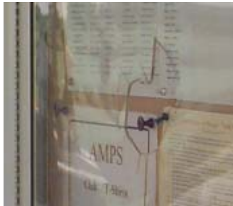
Vandals broke the Plexiglas panels in both doors of our Bulletin Board at the field. Repairs shouldn't be difficult as nothing else was damaged. We plan on using Lexan replacement panels this time.
